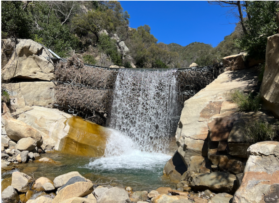
Figure 1: Upper San Ysidro Creek ring net plugged with vegetation and debris - April 1, 2023
